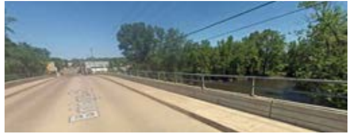
The north side of the Bridge Street bridge (as shown right) in Rockford is planned to accommodate the CRRT route by reworking the concrete decking. If modifications to the bridge deck are not feasible, a new grade-separated pedestrian bridge is proposed.
